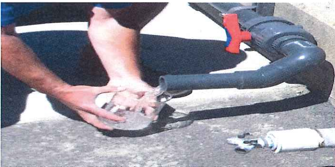
Recycled Water after Filtration and Disinfection
